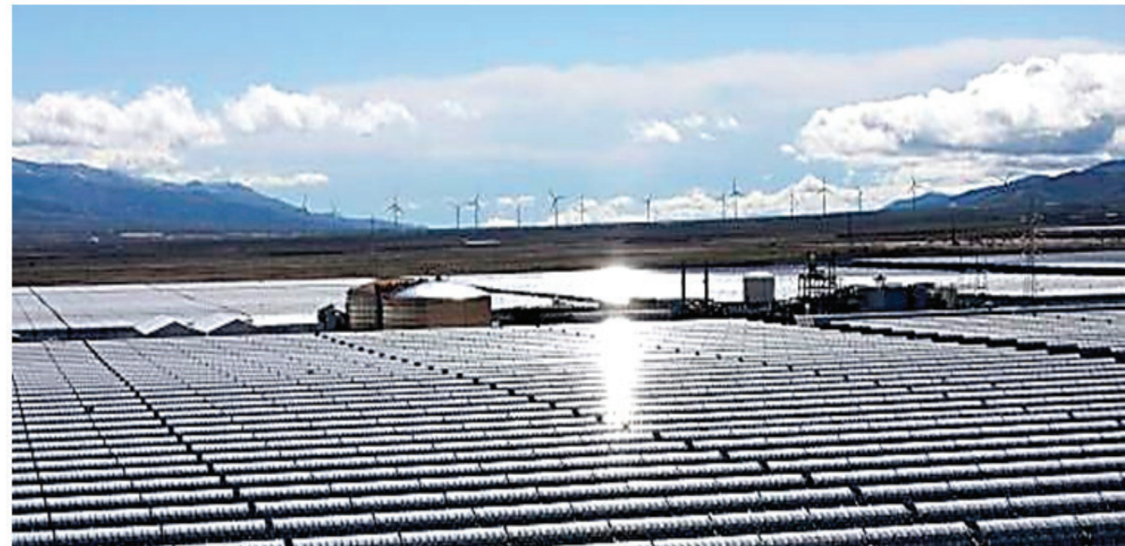
Image: Andasol plants (150 MW) and wind parks (200 MW) in the province of Granada, Spain ©ACS Cobra
